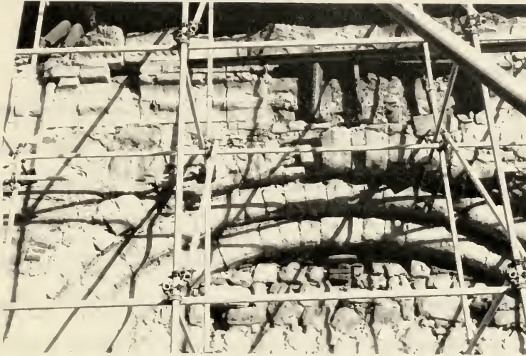
Fig. 14. East wall of nave. Disaggregated and cracking tuff blocks in cornice.
